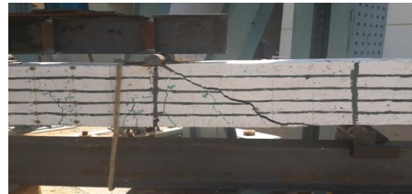
Fig. 17 Failure of GB under flexure
