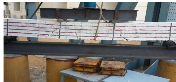
Fig. 18 Failure of SB under flexure
