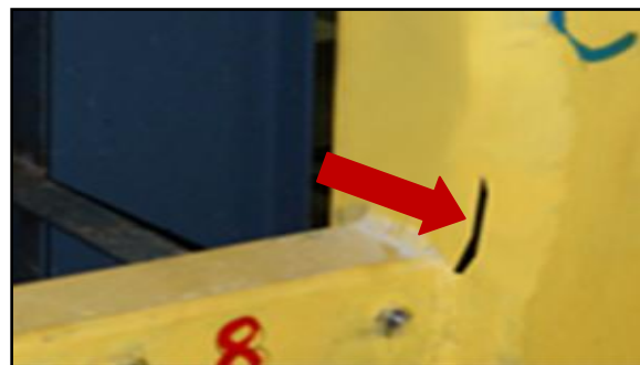
Fig.28 Column Crack at a Base Shear of 80 kN– Frame (2)
